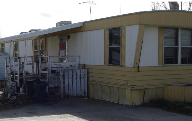
Monitoring the exterior conditions of older manufactured homes is necessary to ensure that certain deteriorated homes are repaired or replaced.
